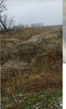
Louisville Access Boat Ramp Site 6 Scour Hole
