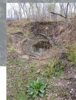
Tyson Bend Wildlife Area Site 3: Scour Hole
